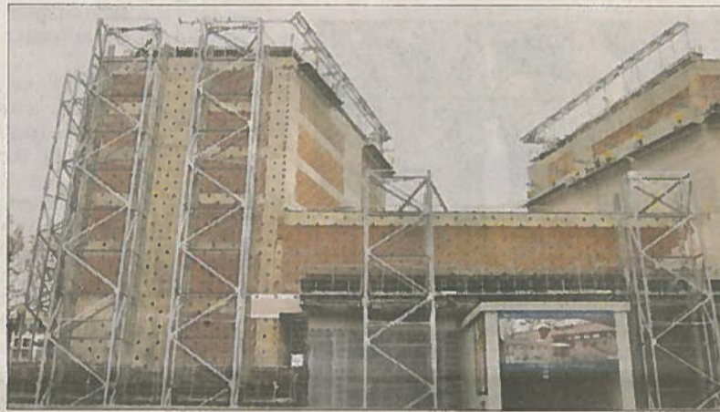
Pablo Garcia, a mason's helper, above, reattaches a marble panel to the National Gallery of Art's East Building, at left. All 17,000 pieces of the building's marble cladding are being removed and reattached to correct a problem with the fastening system.
